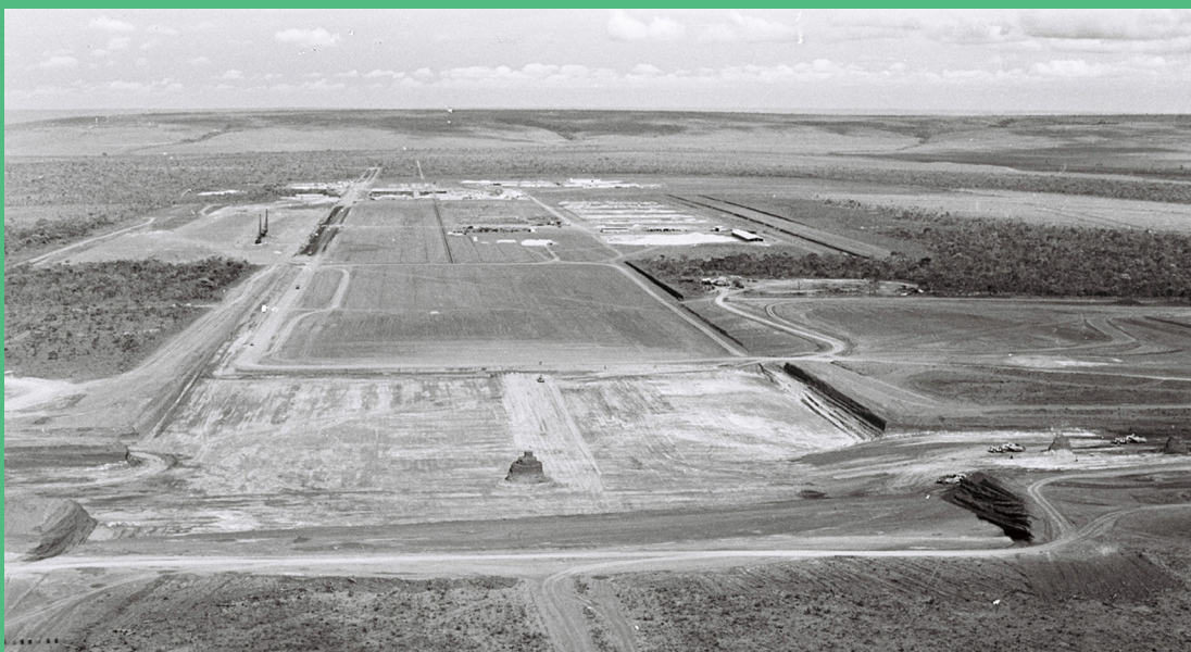
Image 1: An aerial view of the earthworks for the construction of Brasilia, showing the strategy of designing with the ground
